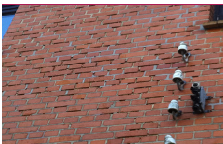
Plasterer bees - joints in masonry partially broken down. (Photo: Protox)
