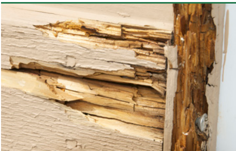
Gilled polypore - degradation in wooden clad- ding in holiday homes. Attack 3-4 years old. (Photo: Protox)
