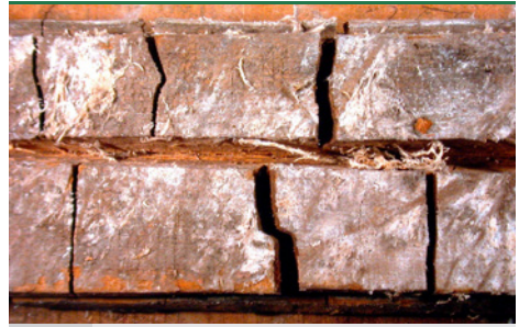
svn 50 Dry rot fungus- crevice blocks. (Photo: Hussvamp Laboratoriet)
