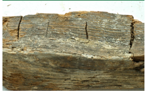
Dry rot fungus - old attack. Weak mycelial remains and clear transverse fissures. (Photo: Protox/Goritas)
