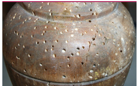
in 17 Common furniture beetles - exit holes in table legs. (Photo: Protox)
