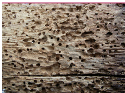
Deathwatch beetle - exit holes in an old beam. (Photo: Protox)
