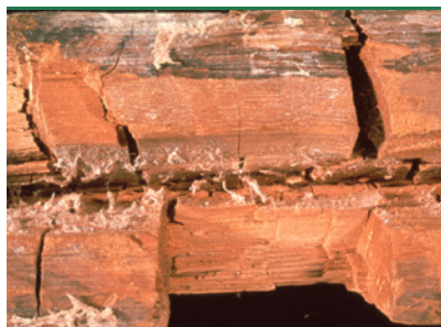
Dry rot fungus- crevice blocks. (Photo: Protax/Gori)
