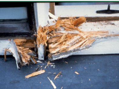
sv 30 Bark fungus (white rot) in the window sill. (Photo: Goritas)
