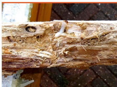
Decayed wood with insect infestation
