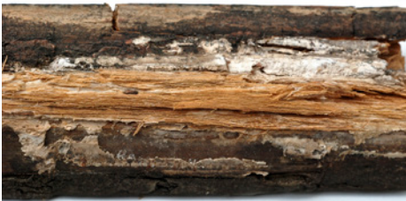
svn 53 Bark fungus in window frame (white rot). (Photo: Goritas)
