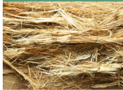
White rot - the fungus breaks down the lignin in the wood, leaving the cellulose threads. This frays the wood.
