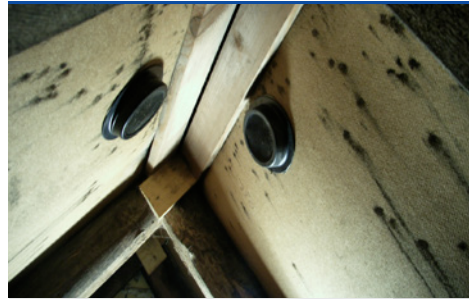
Black mould on the roof due to lack of ventilation of the roof space (valves retrofitted). (Photo: Prottox)
