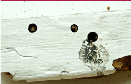
in 14 Red-brown Longhorn Beetle - exit holes in door frame. (Photo: Protox/Goritas)
