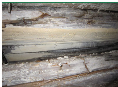
Mine fungus - fruiting bodies, surface mycelium and crevice blocks in floor joists. (Photo: Bøgh & Helstrup)
