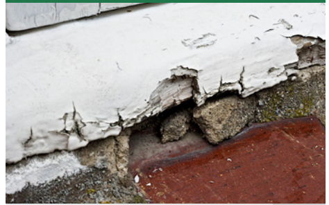
Surface rot (grey rot) - dripping on old window. (Photo: Prottox)
