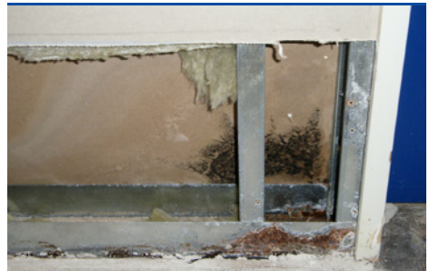
Mould growth ( Stachybotris chartarum ) in light plaster wall after flooding. (Photo: Prottox)
