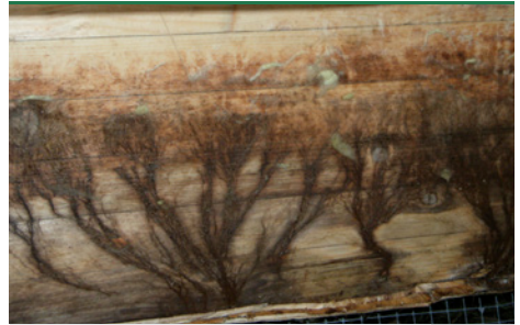
Wet rot fungus - brown stringy mycelium on glulam beam. (Photo: Protox)
