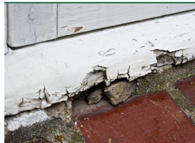
Grey rot (Surface rot) - dripping on old window.
