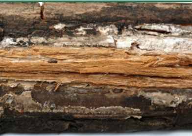
sv 29 Bark fungus (white rot) in window frame. (Photo: Protox)
