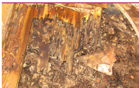
Orange ants - decomposed floorboards. (Photo: Protox/customer photo)
