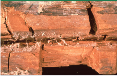
svn 49 Dry rot fungus - broken down wooden beam. Brown rot with large fissure blocks and surface mycelium. (Photo: Protox/Gori)
