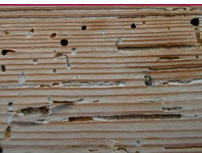
i 11 Common furniture beetles - floorboard with exposed larva passages as a result of planing. (Photo: Prottox)
