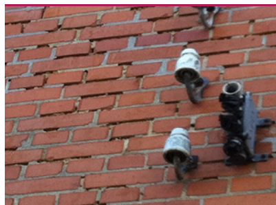
Plasterer bee – broken joints in brick gable. (Photo: Prottox)
