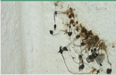
Cellar cup fungus - fruiting body on wall by skirting board. (Photo: Bøgh & Helstrup)
